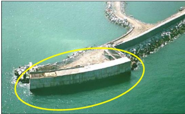
Figure 3. Multi-chamber OWC plant integrated into a breakwater, Spain
