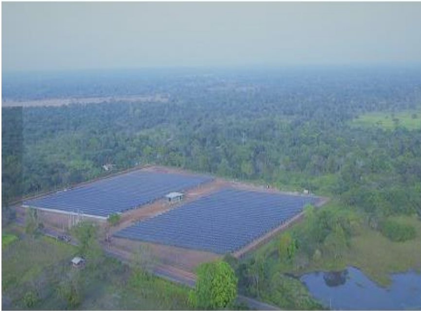
Figure 4.3: Vavuniya Solar Power Station
