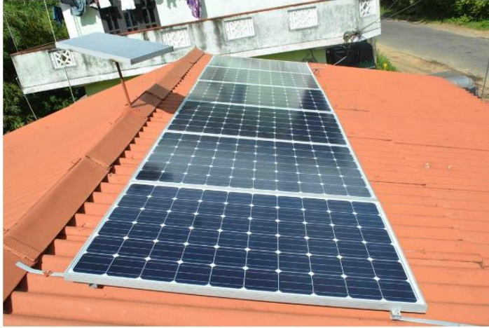
Figure 4.5: Gampola solar power station
