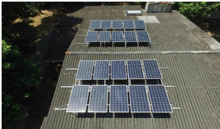
Figure 4.4: Aniwatte solar power station
