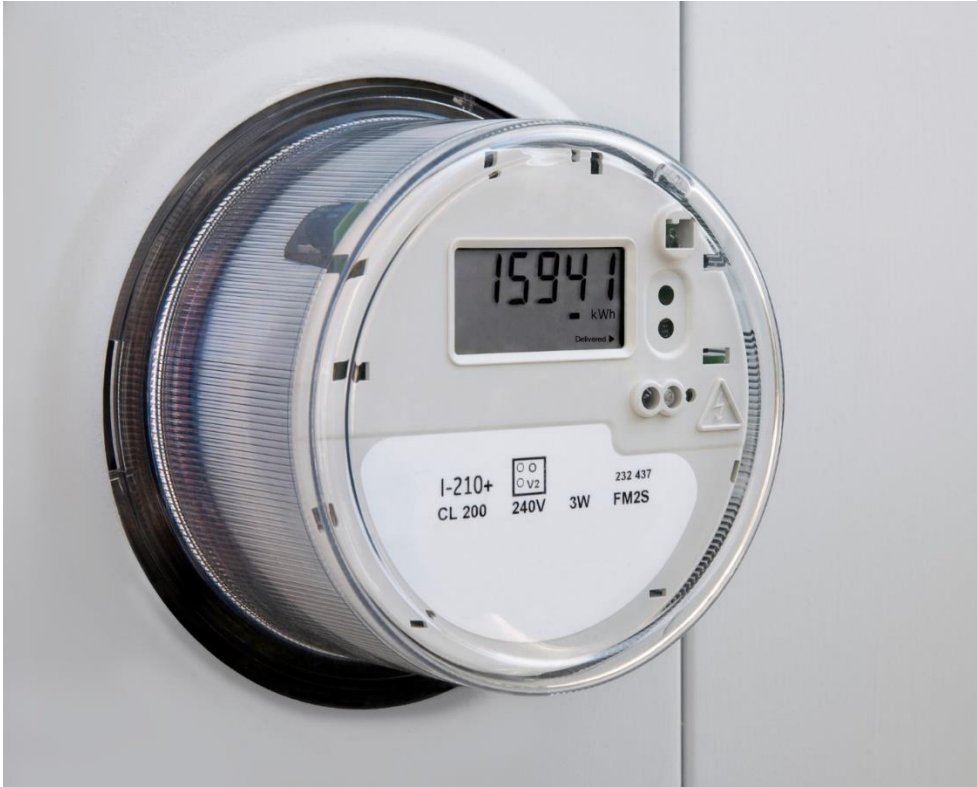
Figure 2.5: A smart electric meter
