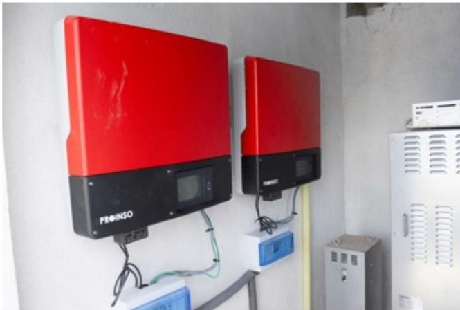
Figure 4.6: Aruppola solar power station
