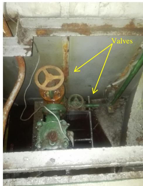
Figure 1: Bad valve placement in OPV-A
