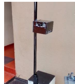
Figure 2. Intruder identification and notification system
